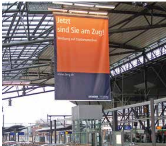
2008 Erfurt railway station Winch for advertising banner
